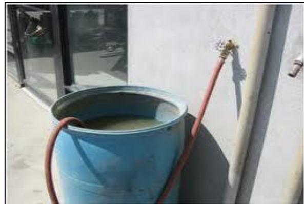
Hose left in a drum filled with contaminated water.
